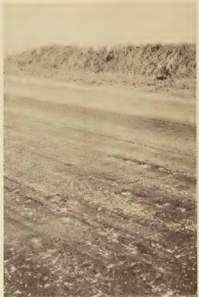
FIGURE 6.—SURFACE WAS PARTLY CRUSTED AND HARDENED AT THE TIME OIL WAS APPLIED. SHRINKAGE CRACKS ARE NUMEROUS AND PITTING IS EVIDENT
